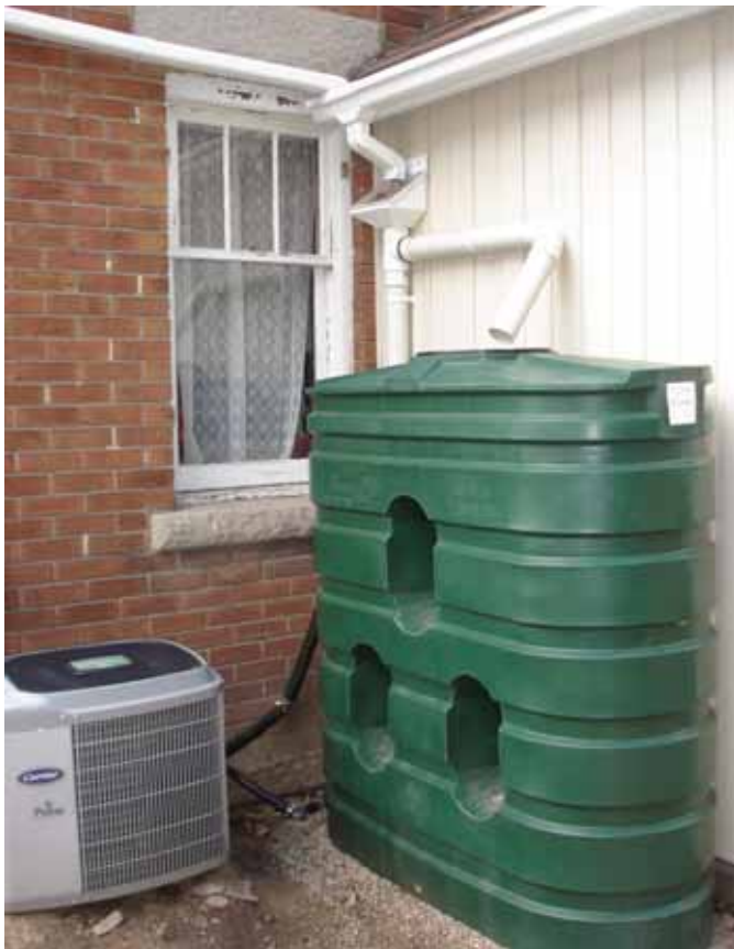
RAINWATER HARVESTING CISTERN
